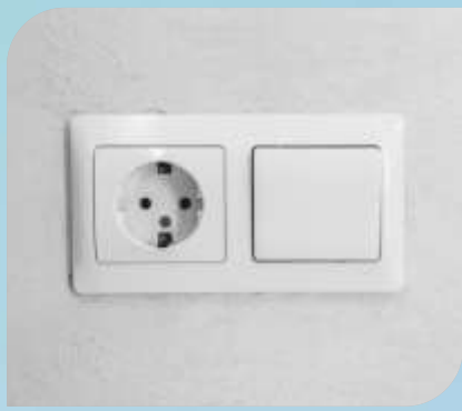
SUFFICIENT ELECTRIFICATION POINTS
