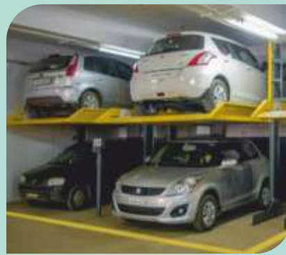
MECHANIZED CAR PARKING
