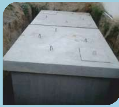
UNDERGROUND & OVERHEAD WATER TANKS
