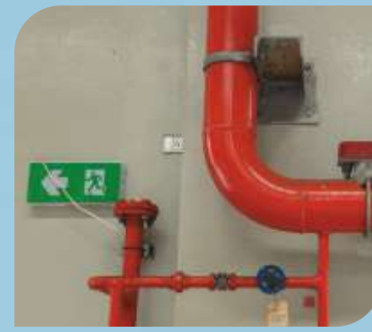
FIRE-FIGHTING SYSTEMS WITH ALL FITTINGS
